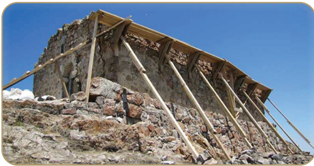
During the occupation, illegal repairs were conducted to the temple, and the roof was built with completely modern materials
